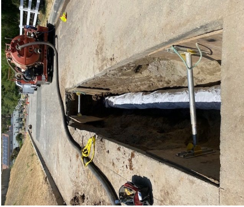
Above is a repair attempt in June 2023
