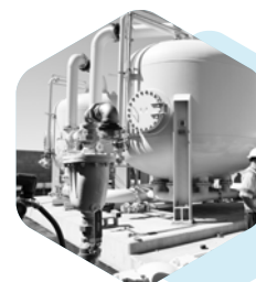
VALLEY CENTER WELL TREATMENT FACILITY
