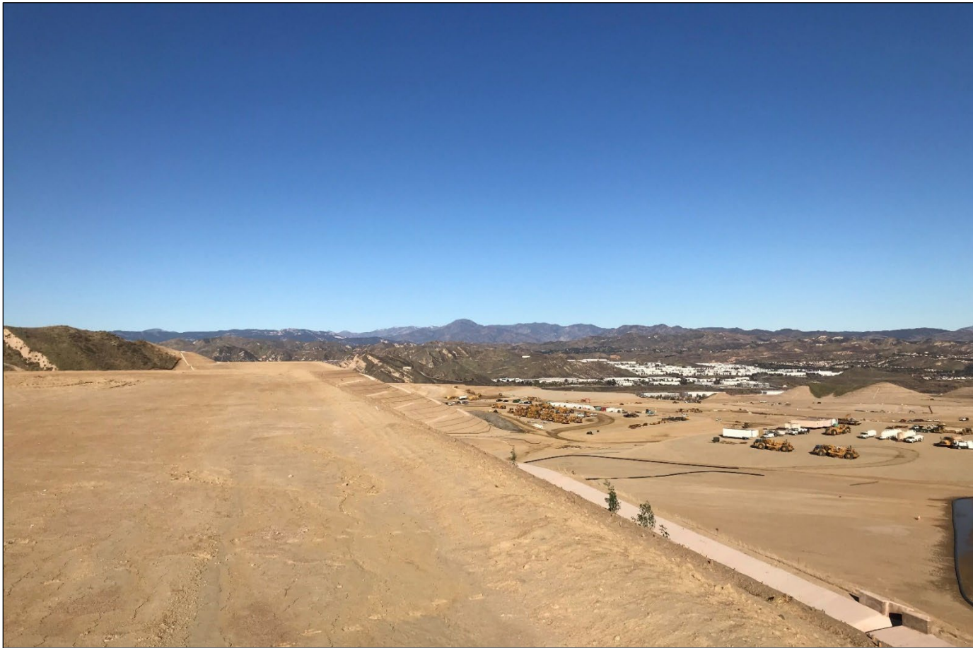
Backcountry Reservoir site facing northeast, with grading for Mission Village development taking place on the east.
