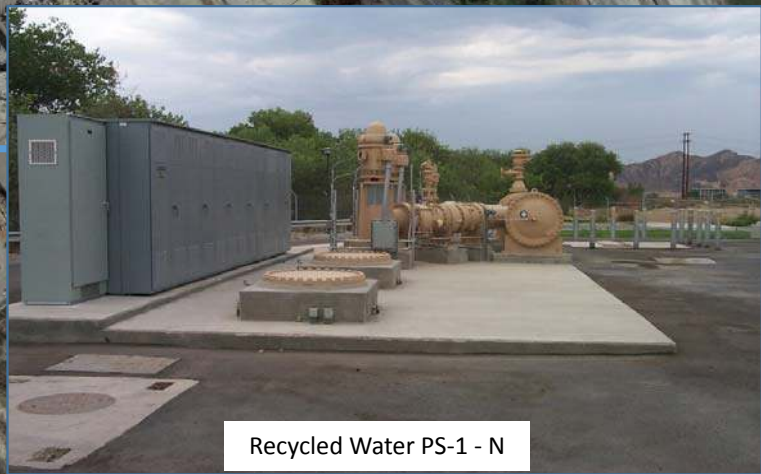
Recycled Water PS-1 - W
