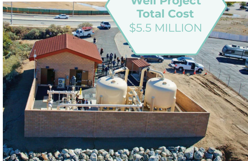
VALLEY CENTER WELL TREATMENT FACILITY
