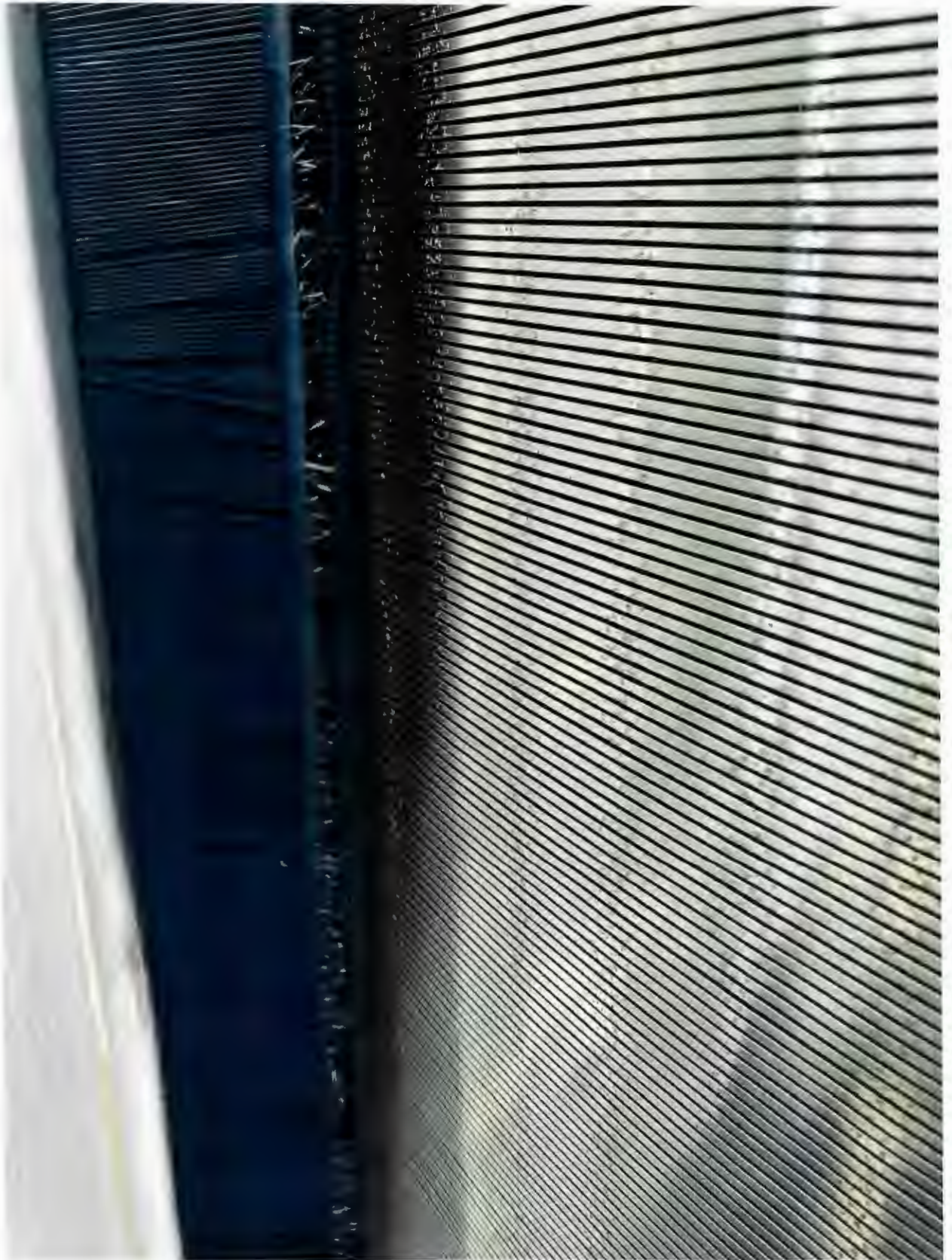
Nylon brush used to periodically clean screens
