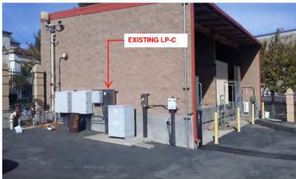
Figure 1.2.3 – Existing Lighting Panel (LP-C) located at Chemical Storage Building
