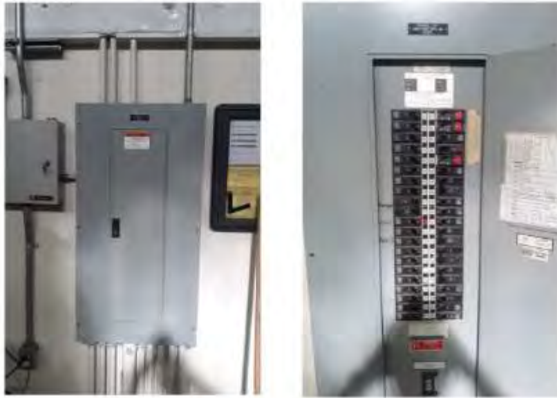
Figure 1.2.2 – Existing Lighting Panel (LP-A) located at the Pump Room
