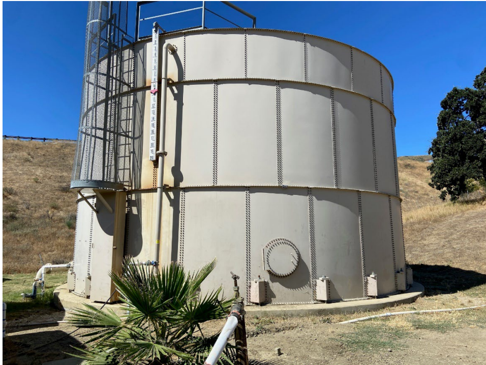
On-Site Water Tank
