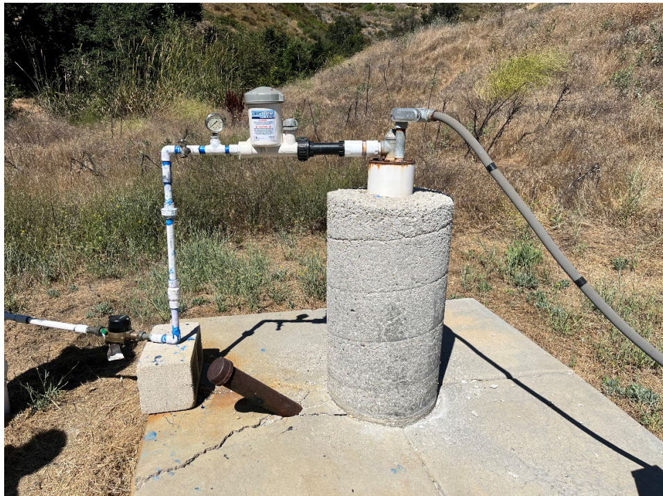
One of Five On-Site Water Wells
