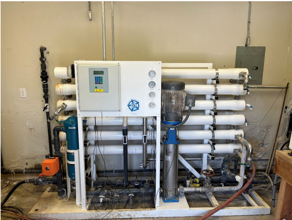
On-Site Reverse Osmosis Well Treatment System
