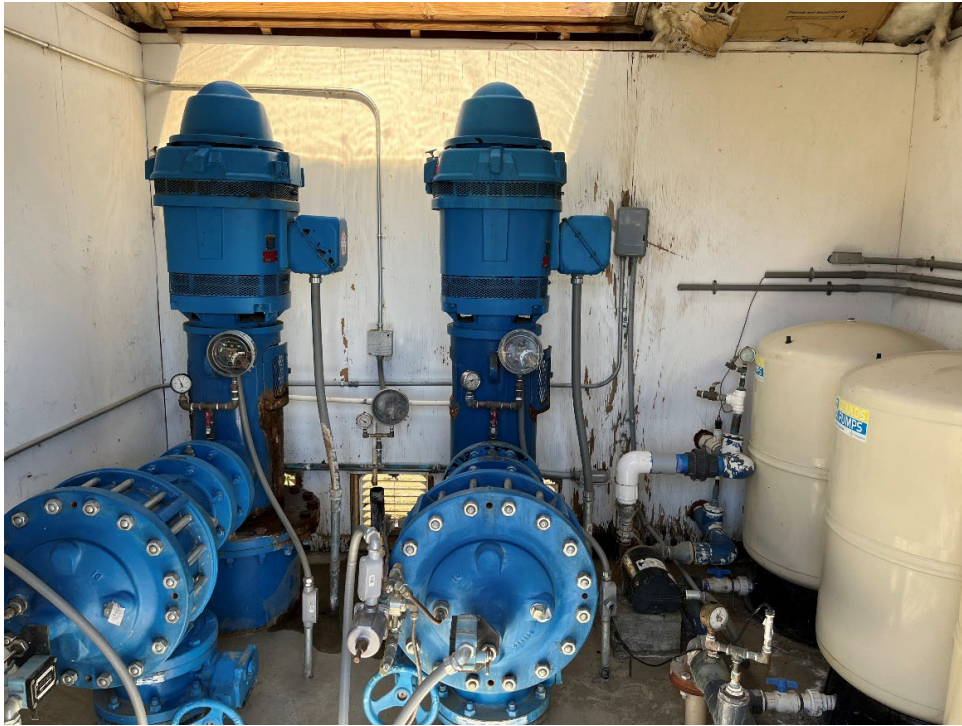
On-Site Pumping System
