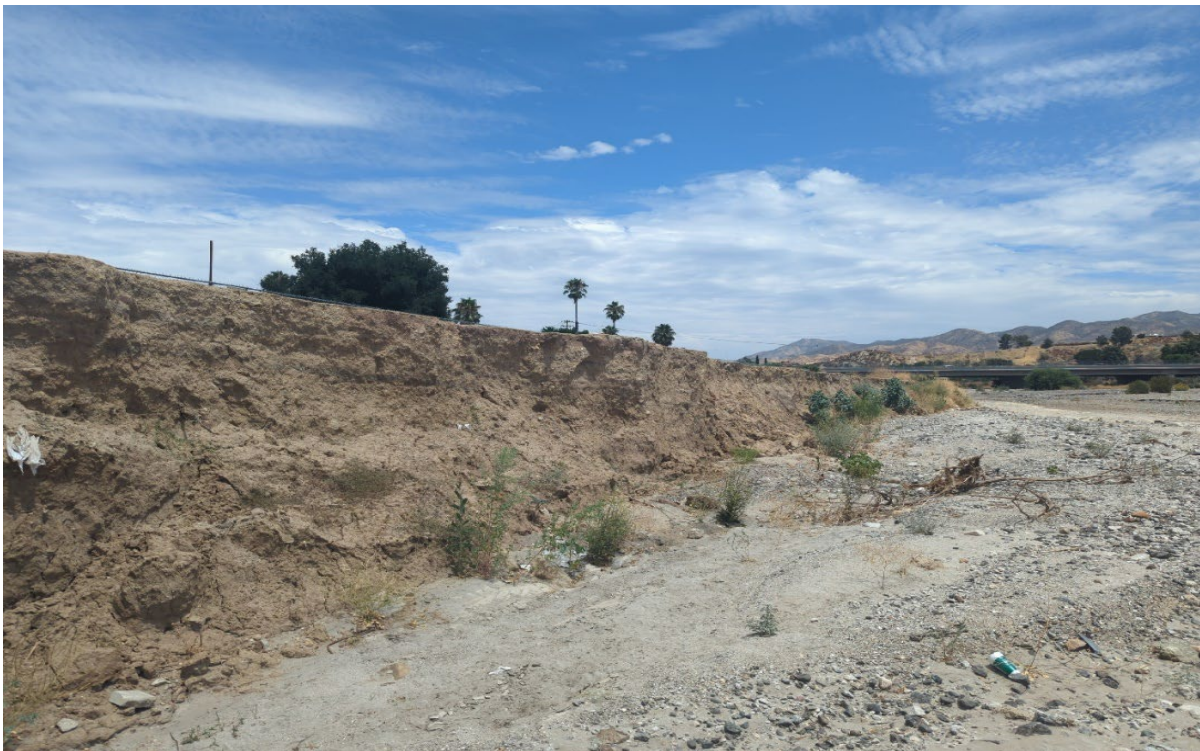
Photograph 18. Photo Point 18. View of the northern bank of the SCR in the central portion of the APE where soil cement bank protection is proposed, facing east. Note unstable, eroding bank (August 1, 2023).
