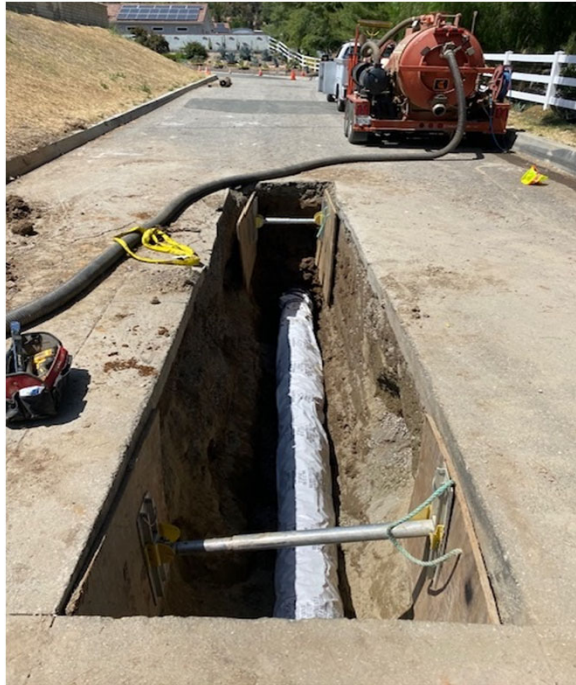
Above is a repair attempt in June 2023
