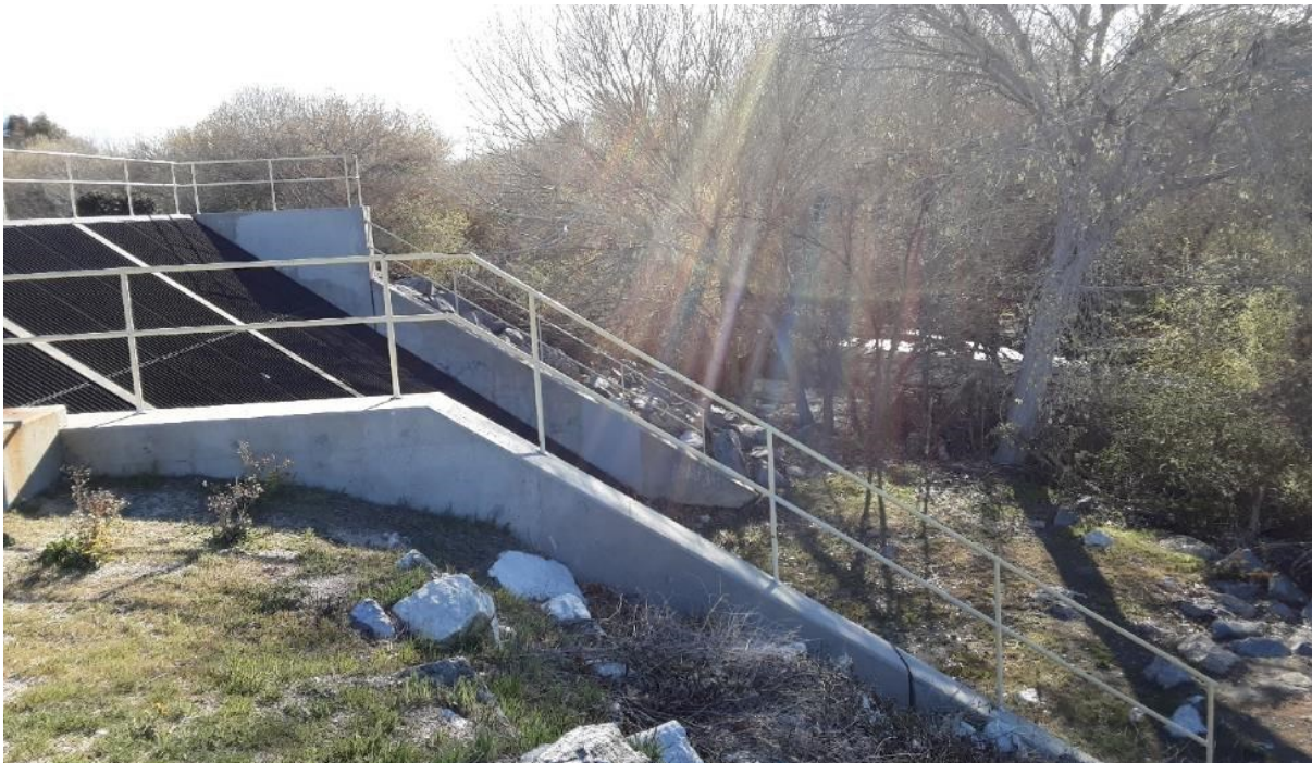
Photograph 6. Photo Point 6. View of the existing concrete outfall structure to the southeast of the Study Area, facing southeast (February 23, 2022).
