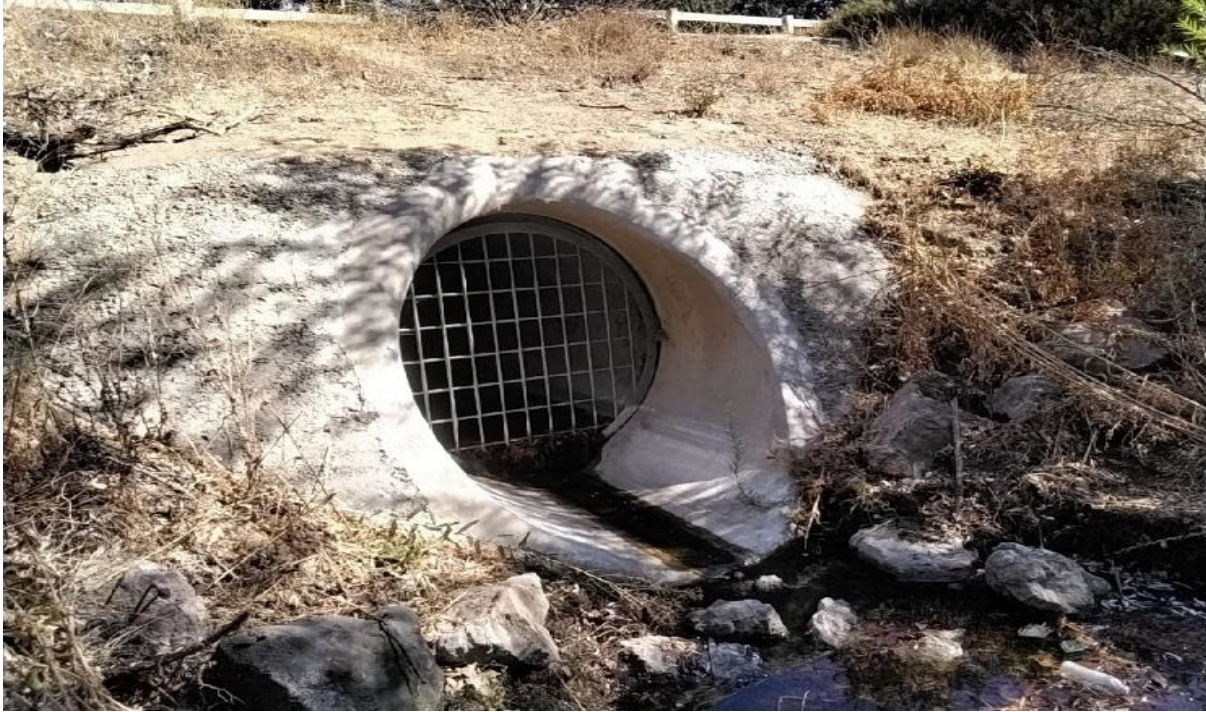
Photograph 29. View of Culvert Outlet 2 in the southern portion of the Study Area, facing northeast (August 30, 2022).
