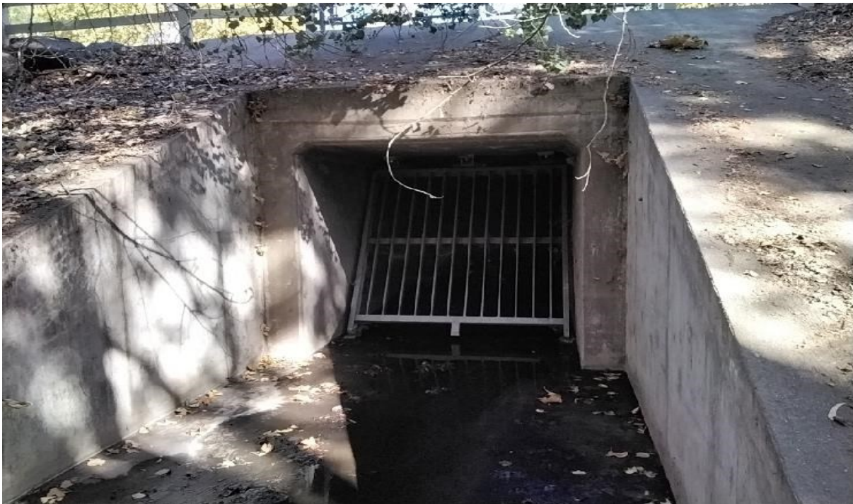
Photograph 30. View of Culvert Outlet 3 along the southern border of the Study Area, facing north (August 30, 2022).
