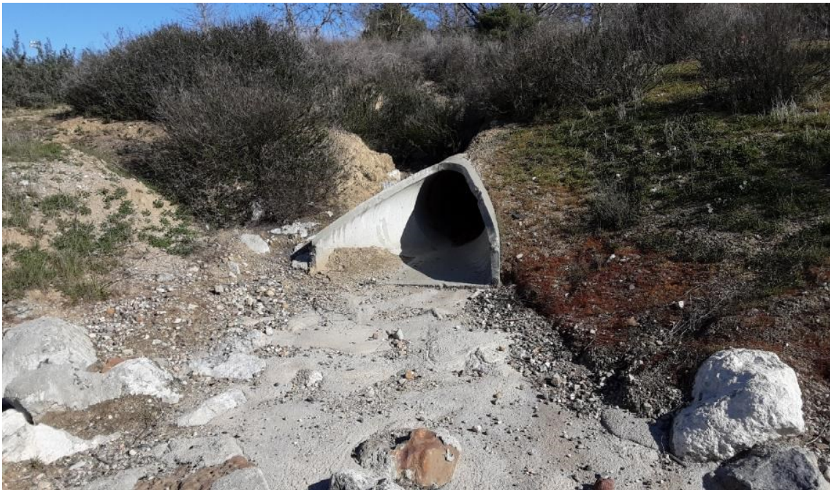
Photograph 10. Photo Point 10. View of Culvert Outlet 1 in the southern portion of the Study Area, facing northwest. Note concrete rip rap to the south (below) the outlet (February 23, 2022).
