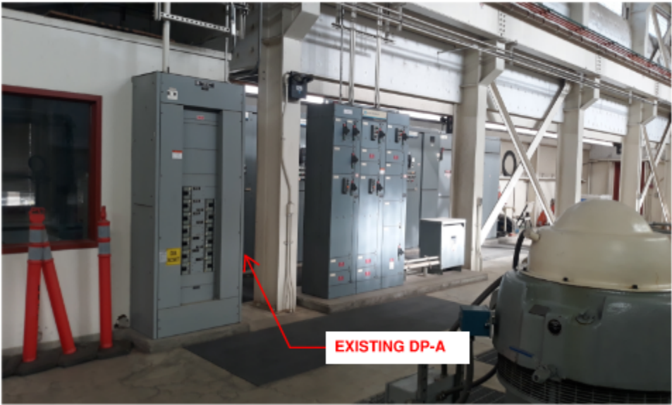
Figure 1.2.4 – Existing Power Distribution Panel (DP-A) located at the Pump Room
