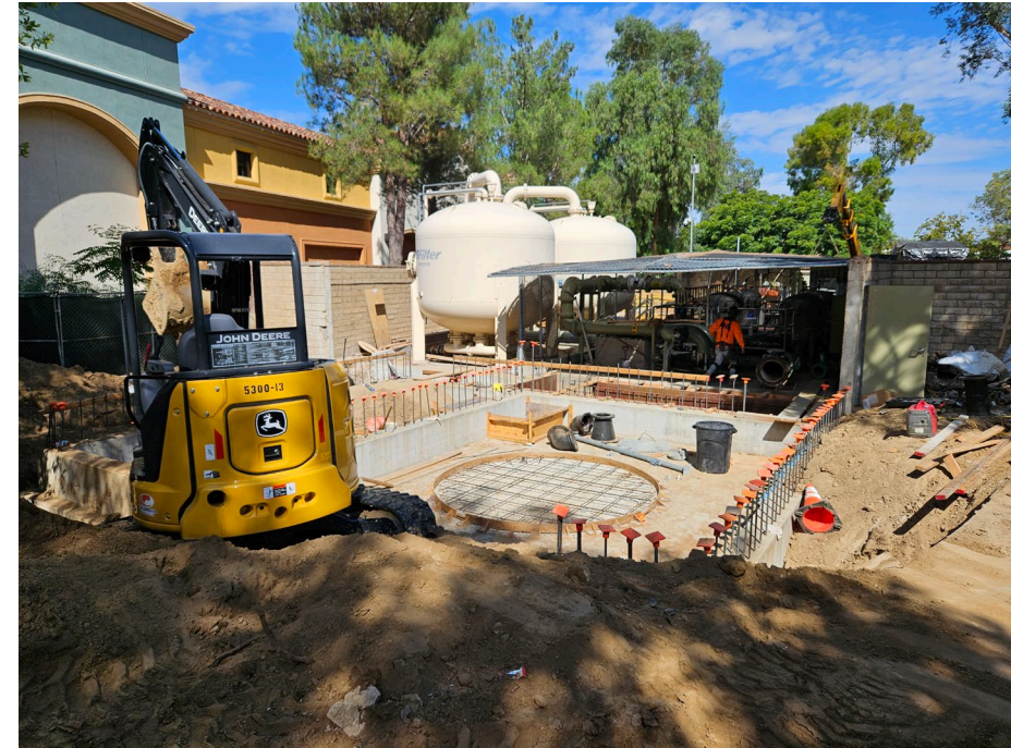
Sodium Hypochlorite Tank Pad
