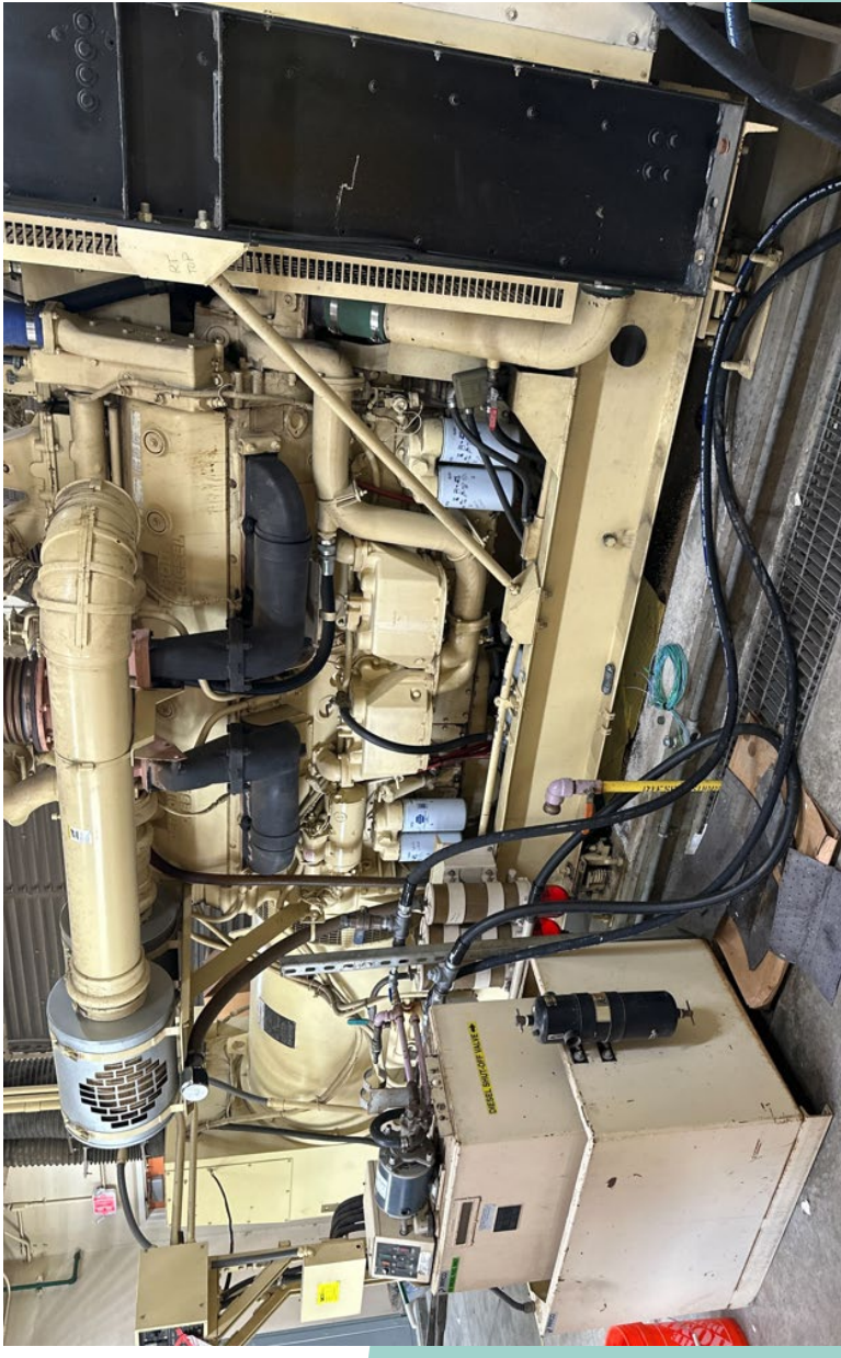
Photo (above): Generator day tank temporarily relocated to avoid timely and unplanned emergency generator outages
